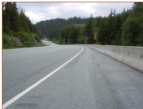
Figure 4.10 – Signed Bike Route with Buffered Paved Shoulder (Rumble Strip), Sea to Sky Highway
